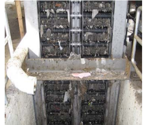
Screens remove debris from sewage at the Headworks
