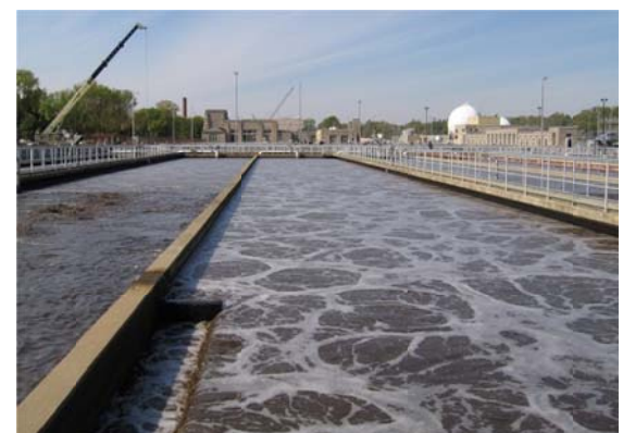
Air bubbles through sewage feeding the “bugs” in the aeration tanks
