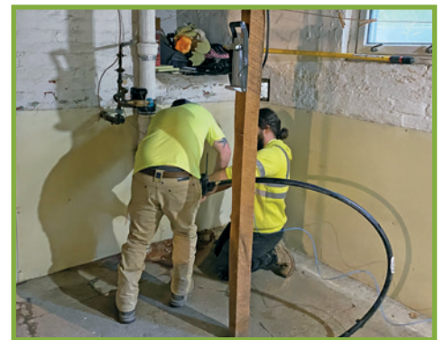
Lead line replacement is connected to the home's meter
