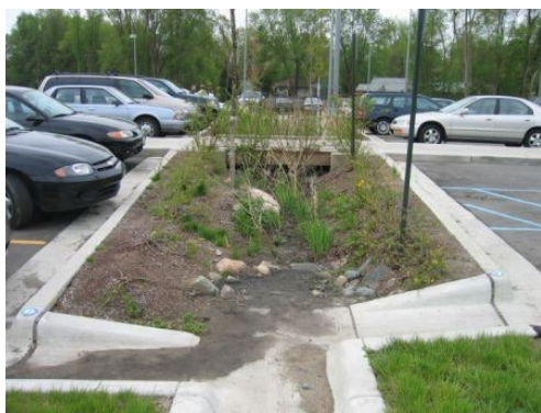
The bioretention area in this parking lot island has accumulated sediment which requires removal.
