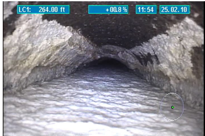
Fats, oils, and grease build-up in sewer main line.
