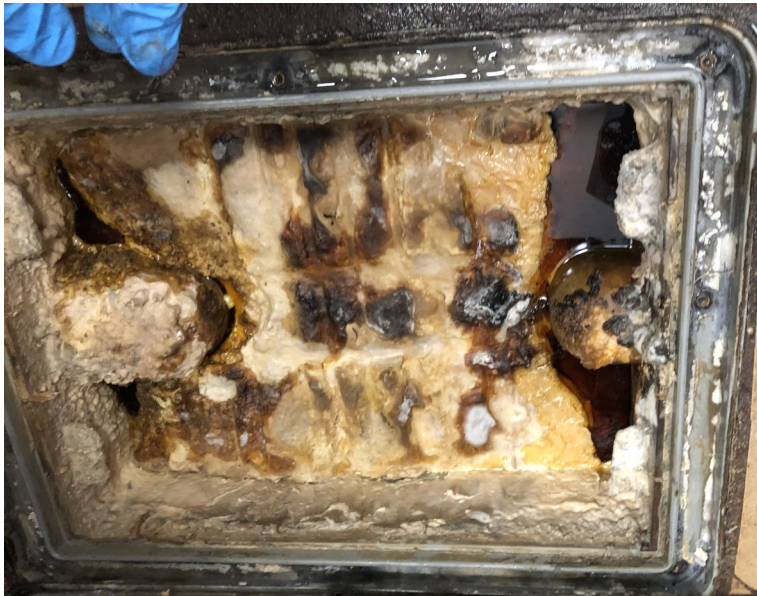
Grease trap that was not properly maintained
