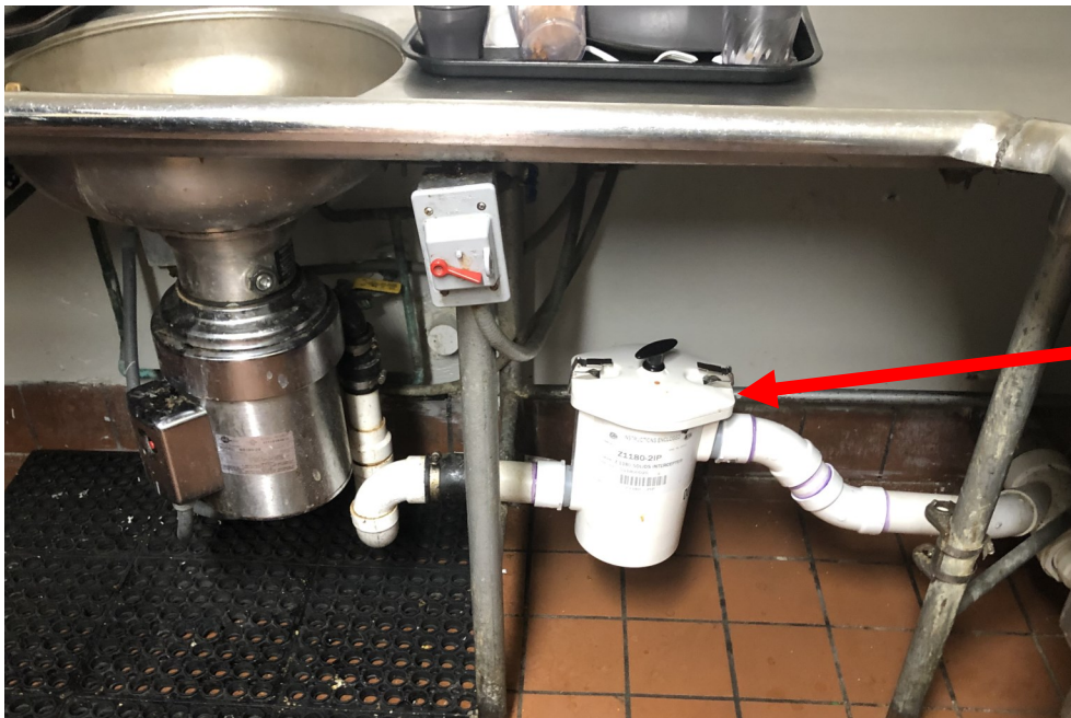
Solids interceptor/ separator installed after garbage disposal
