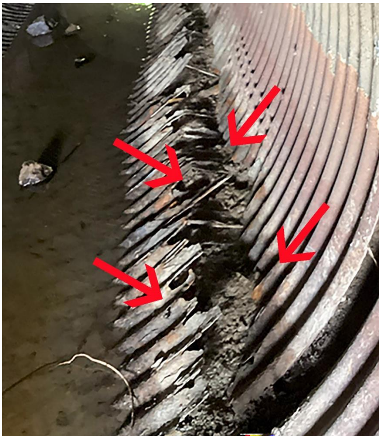
Photo showing the deteriorated condition of a large-diameter culvert pipe under Adams Center Road. The bottom right area and a close-up view, marked by arrows, show metal that has worn completely through, with soil entering the pipe as it begins to collapse.
