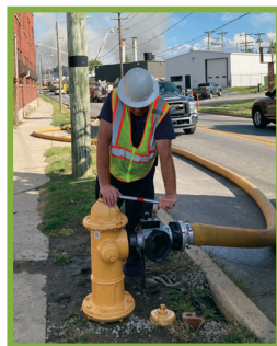
Our Field Operations team maintains 12,240 fire hydrants.
