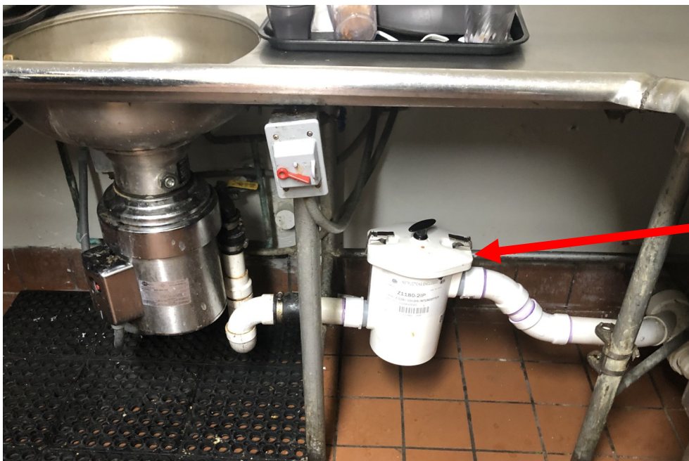
Solids interceptor/ separator installed after garbage disposal
