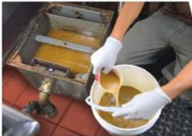
Employee cleaning grease trap
