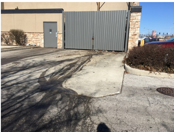
Leaking dumpster area
