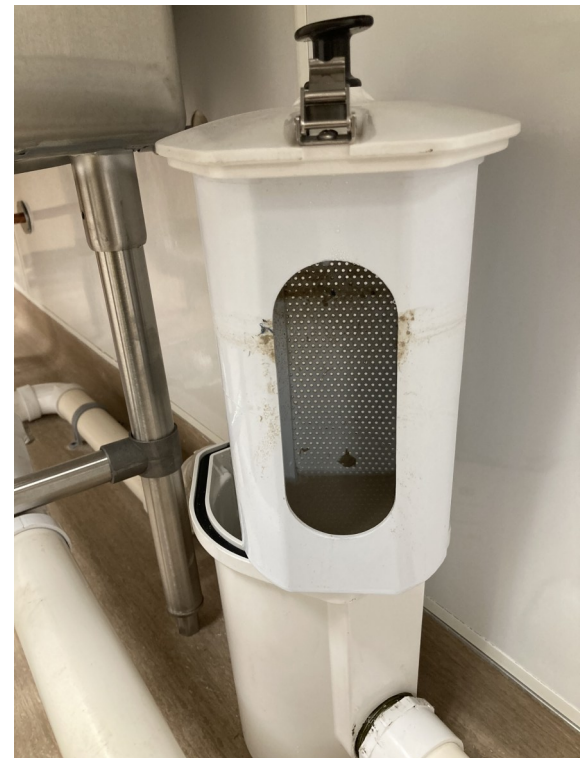
Side view of removed basket
