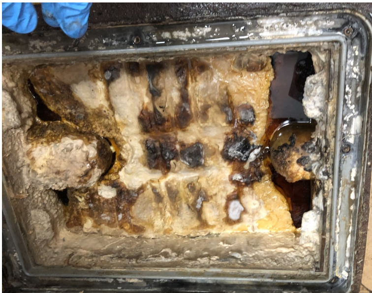
Grease trap that was not properly maintained
